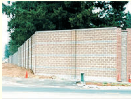
Sound Barrier, Vancouver, WA
